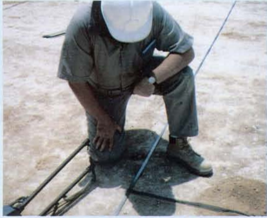
Mixed Metal Oxide tank base Grid System-connection between anode and conductor bar
